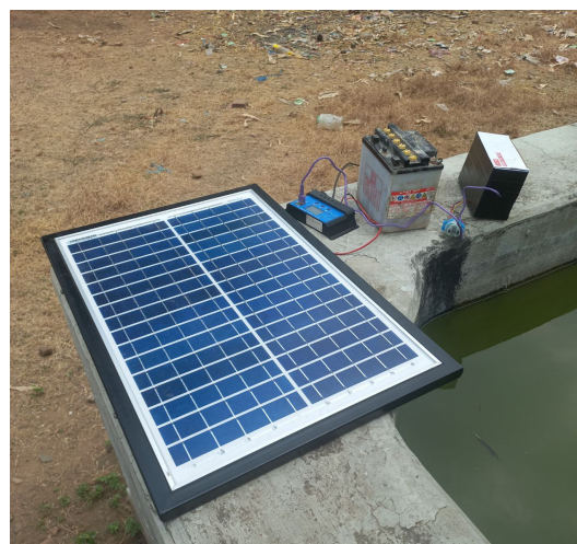
Gambar 4. Alat Monitoring Water Turbidity Berbasis PLTS
